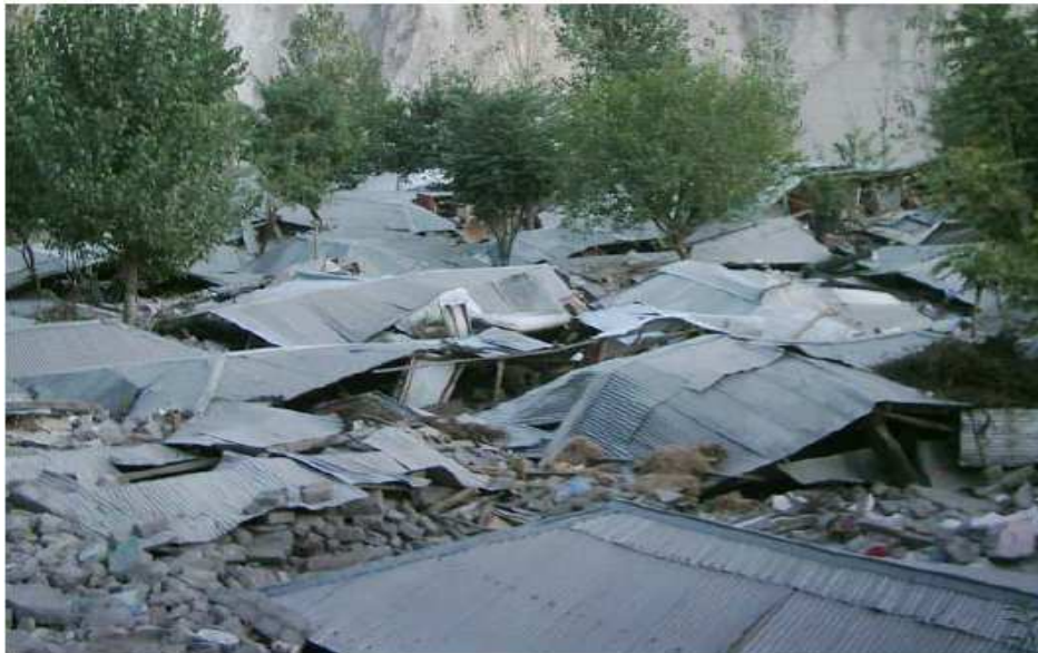
Figure 4: Collapse of unreinforced concrete block masonry houses in Kamsar near Muzaffarabad (Latitude N34° 24.6' and Longitude E73° 28.5')
