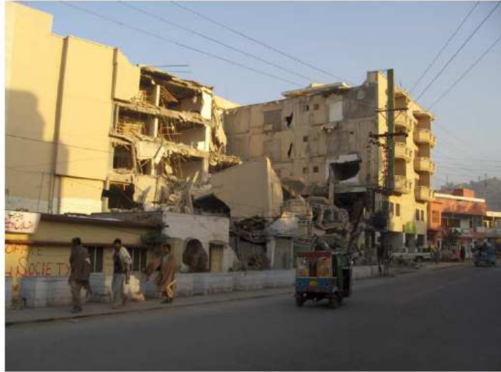
Figure 6: Collapse of Sangam Hotel, a 5 story RC frame building in Domel, Muzaffarabad (Latitude N34° 21.3' Longitude E73° 28.3')
